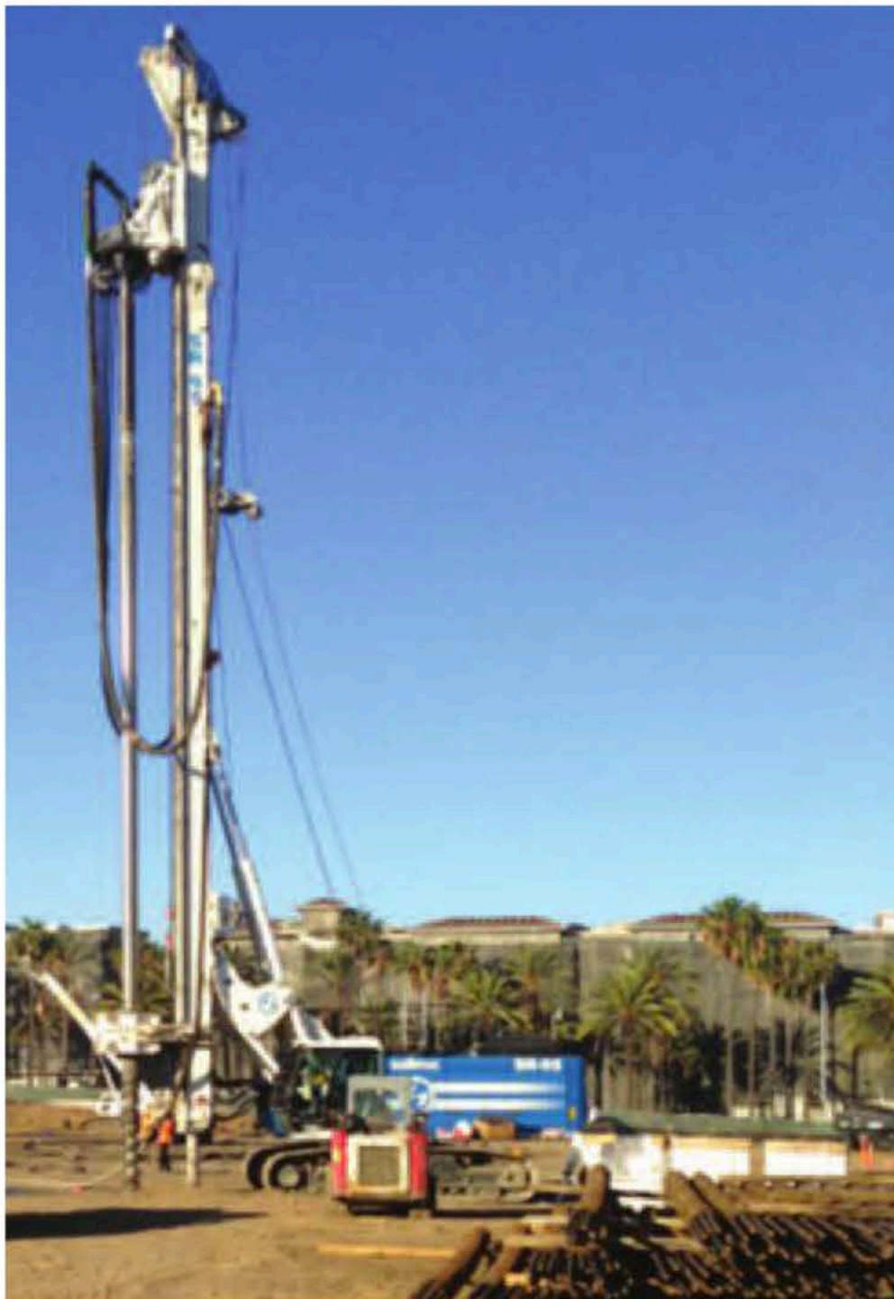
Soilmec SR-95 with Conical Displacement Tooling on a project in California. (Photo courtesy of Condon-Johnson & Associates)
