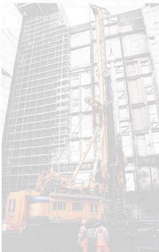
Bauer will lay 600 foundation piles with a diameter of up to 2m and a depth of 60m around the Battersea Power Station in London, UK
