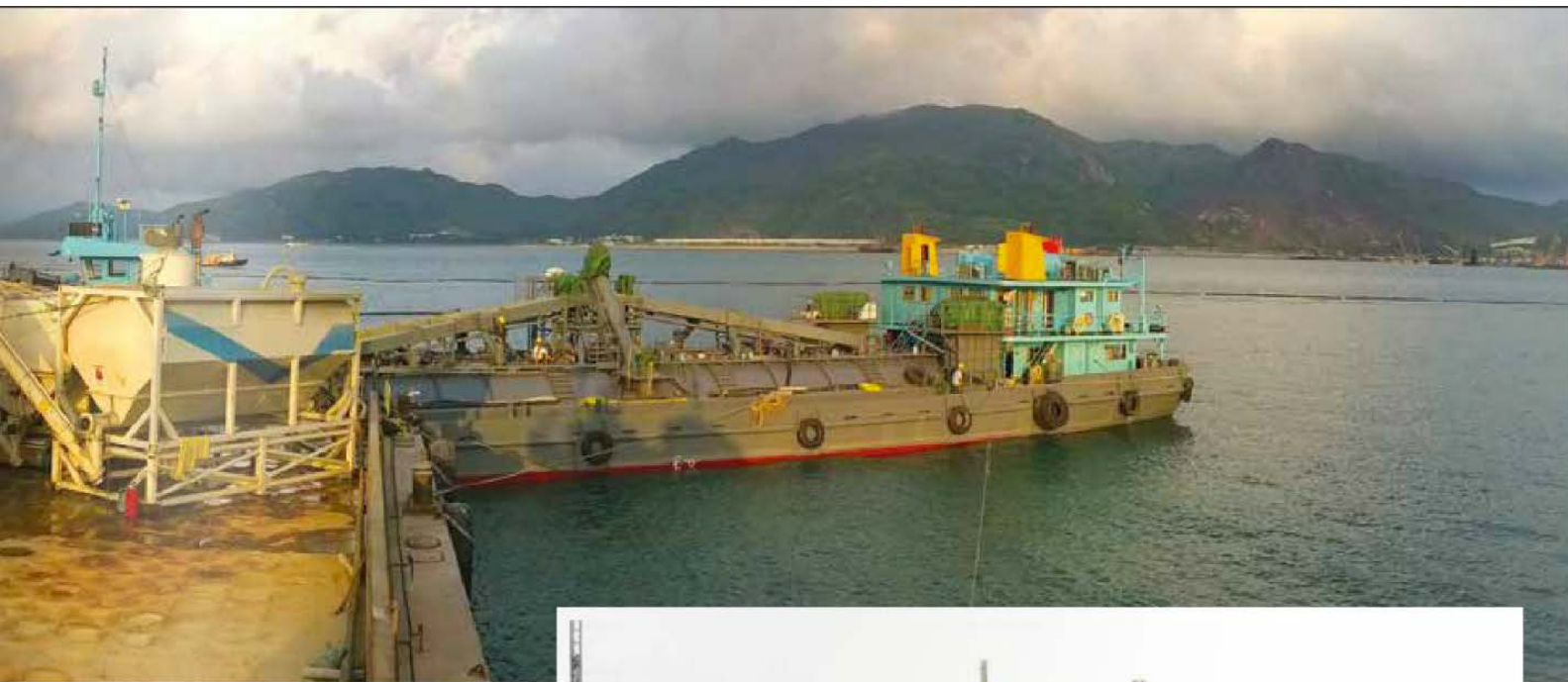
Above: Constructing jet grout columns on an island had its unique challenges, including needing four barges to deliver cement from the factory in China to the jobsite.
