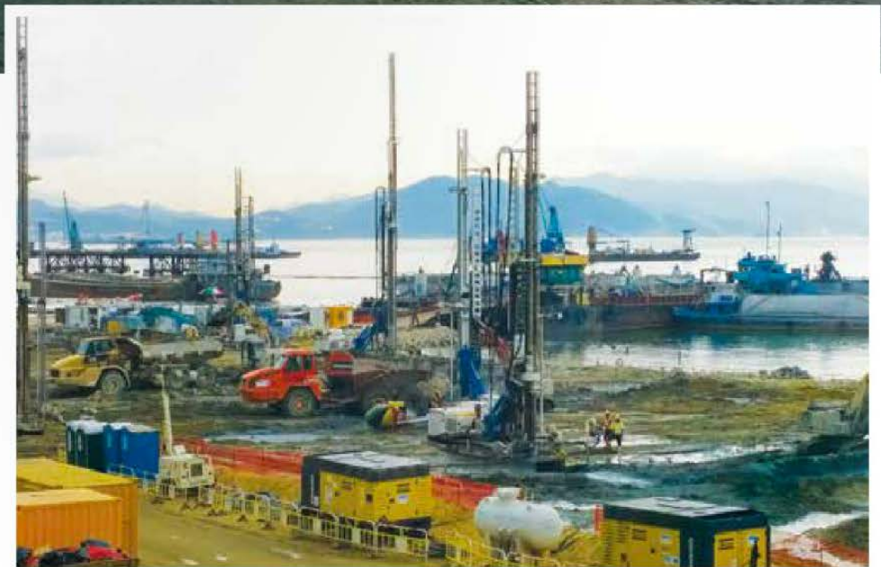
Right: Trevi Hong Kong complete the jet grouting construction in only two months, thanks in part to the reliability of their six Soilmec drilling rigs.
