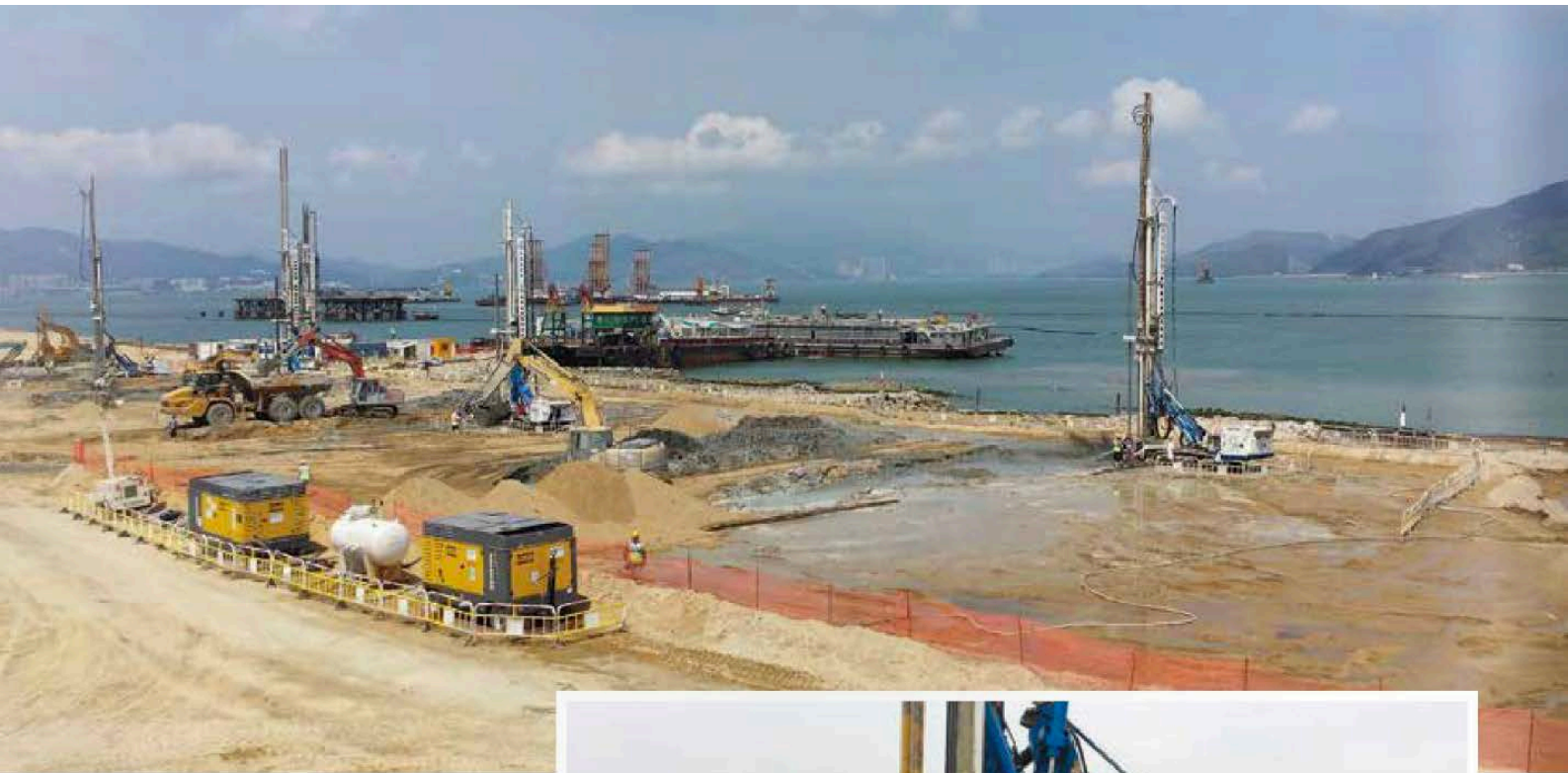
Soilmec PSM-20 rigs jet grouting on an artificial island just northeast of Hong Kong International Airport.
