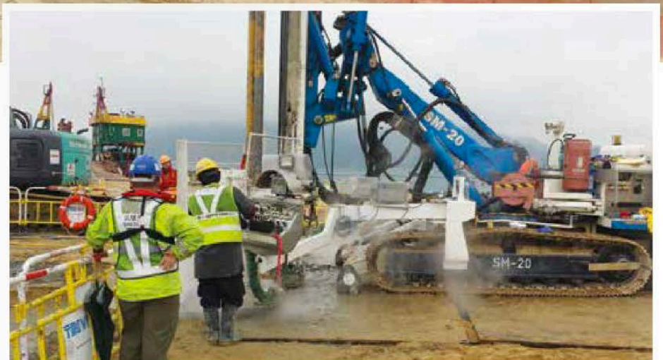
Trevi Hong Kong depended on Soilmec drilling rigs to install 450 jet grout columns, helping to stabilize an artificial island at the centre of the Hong Kong-Zhuhai-Macao Bridge project.
