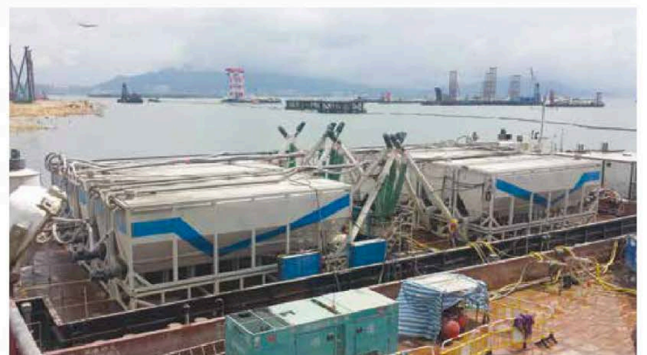
Parked alongside the island, two barges were equipped with 14 silos and four grout mixing plants to keep up with the high consumption rate of cement grout – 1,200 cubic metres per day.
