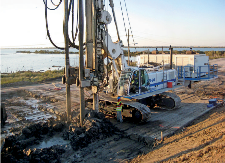
A double axis machine conducts deep mixing for buttresses in an LVP111 foundation (credit, Trevicos)
